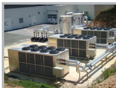
high capacity process chillers
